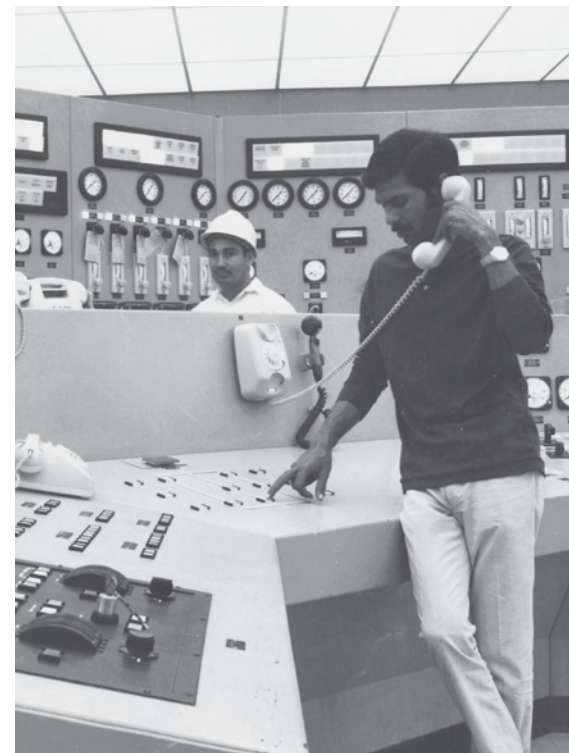
RAPS I control room
